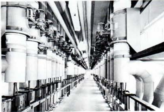
Pent-house installation of Sheldon's PVC Bifurc Fans used for exhausting fumes from Chemistry laboratories at large University.
